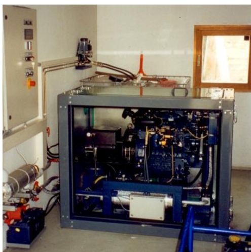
Figure 6: Alpine helicopter rapeseed oil fuel transport for adapted plant oil co-generation at Stüdl hut
